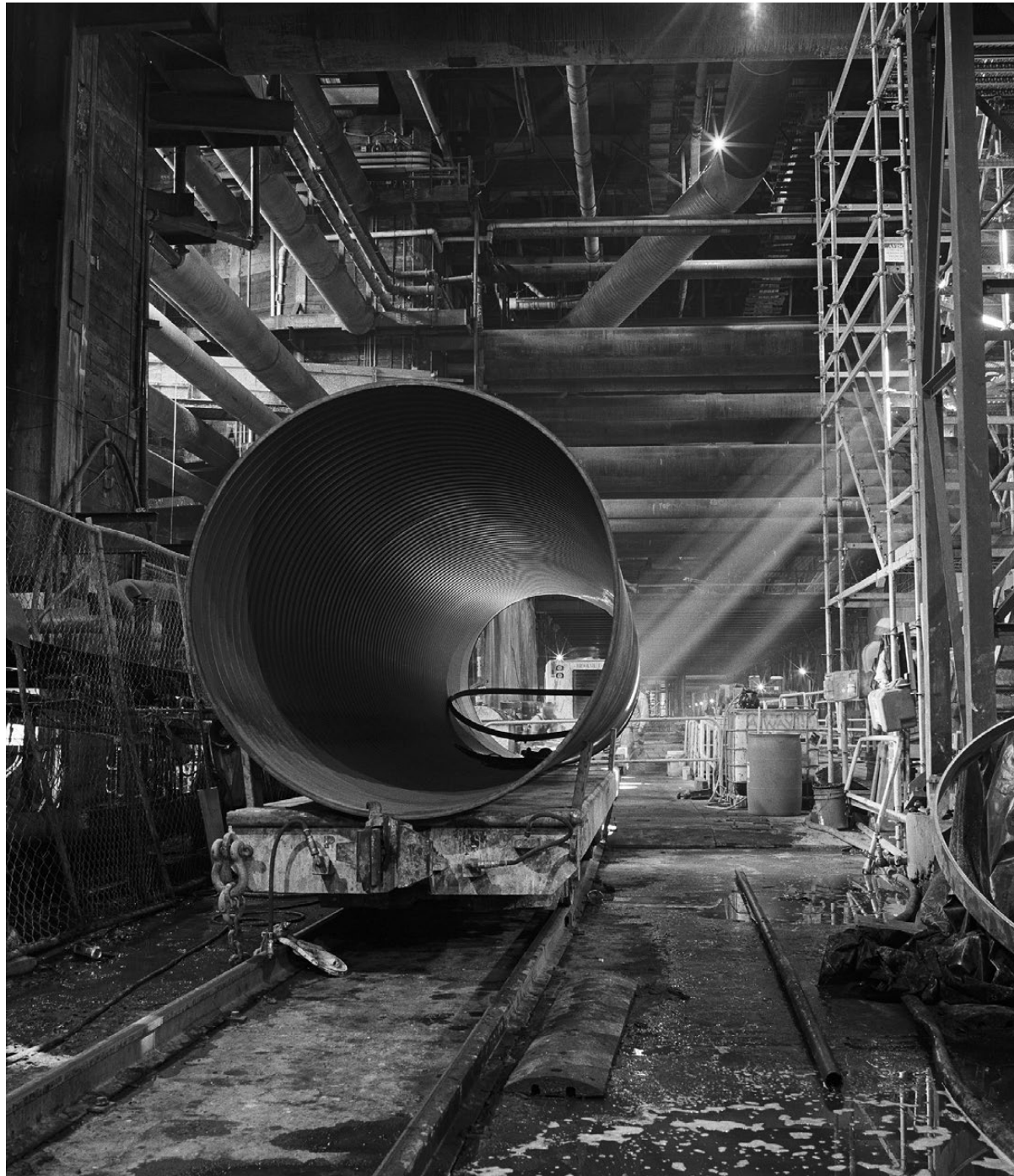
Sunlight filters into the bottom landing at the future station, where a section of air duct waits for transport into a tunnel. As the TBM advances, workers add air ducts, rail tracks and utilities, such as water and power.
