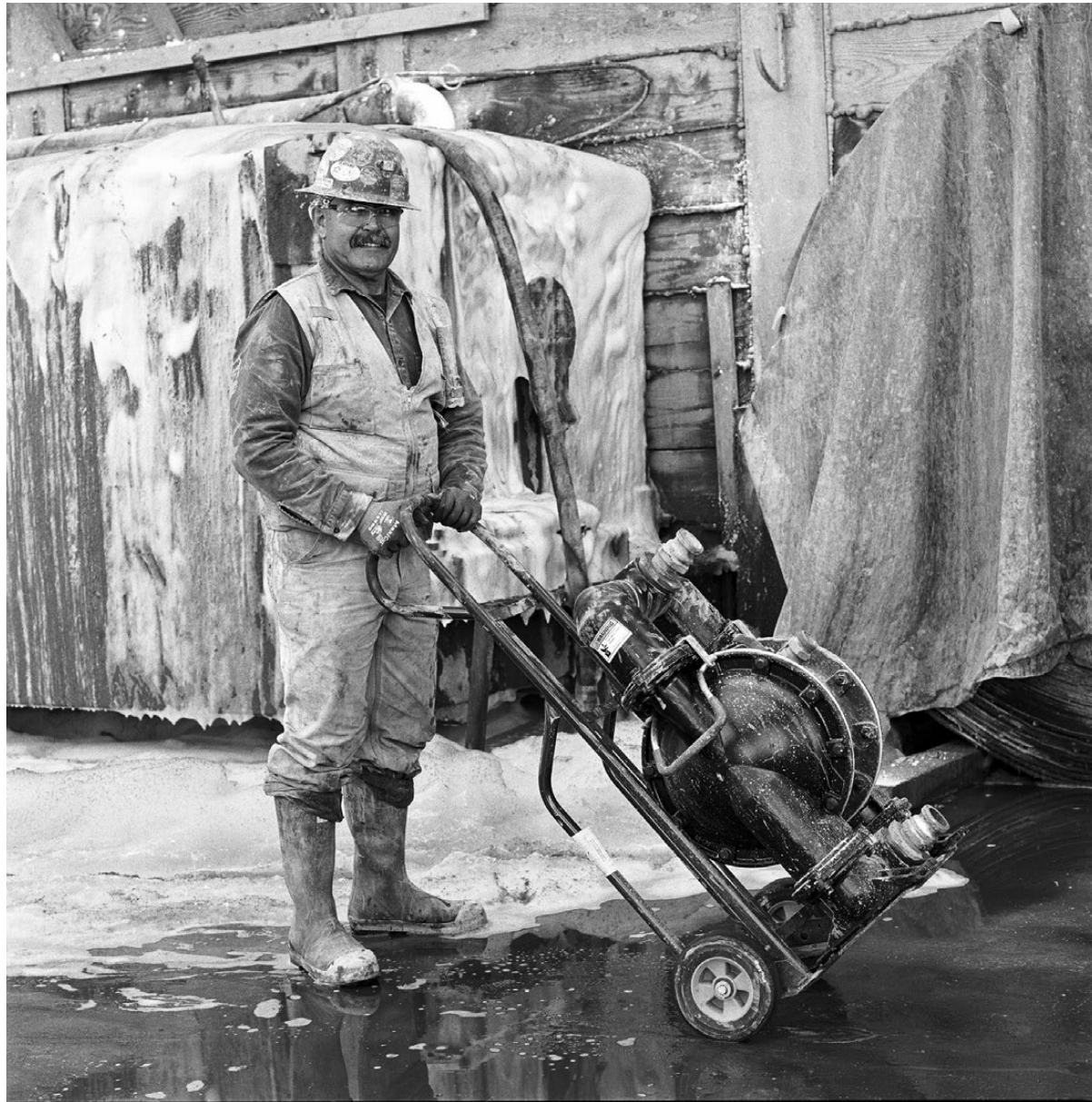
Pompeyo Hernandez, Miner, moves portable water pumps on the topside (above ground). Karagozian shares that Hernandez has worked on Metro's Regional Connector, Purple Line and Red Line.
