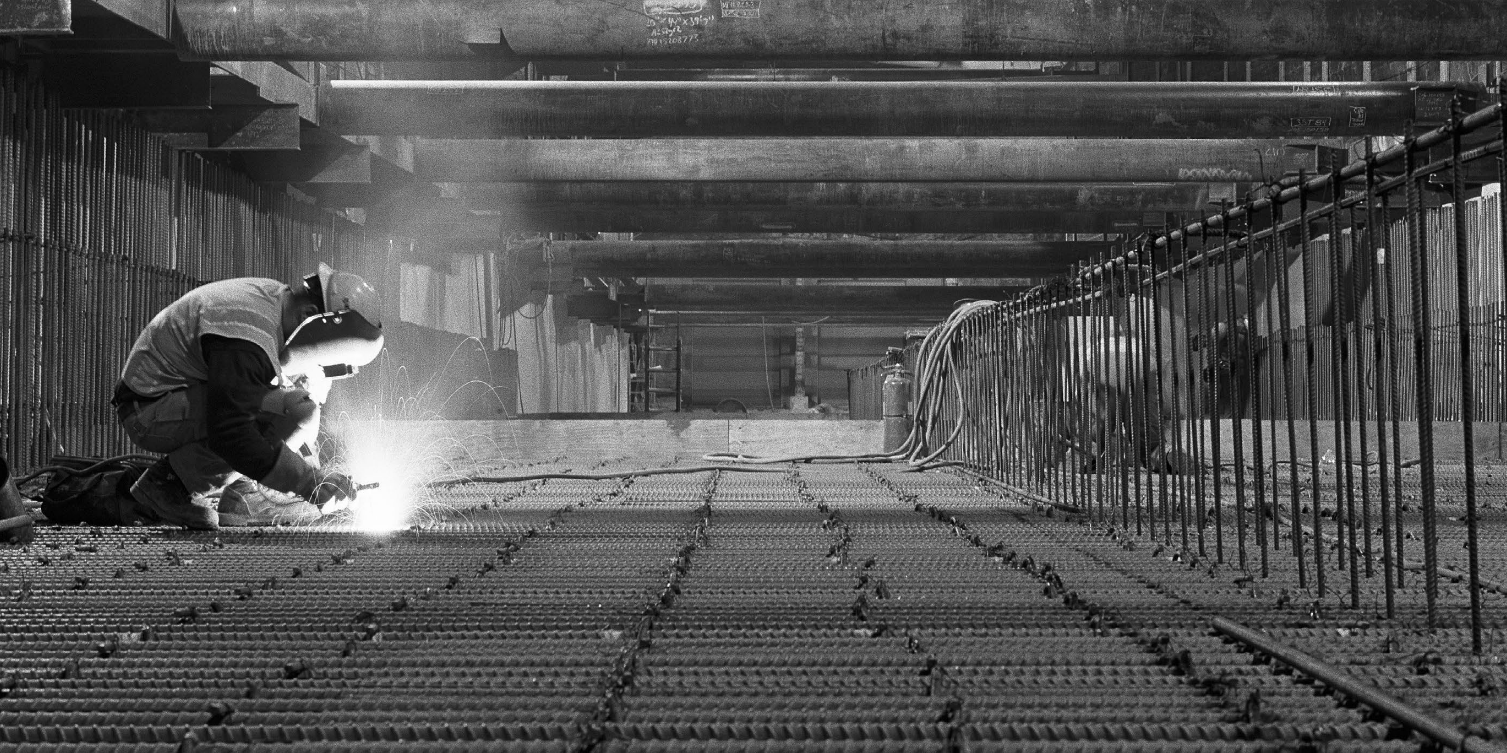
A welder forms the base level of the tunnel box running beneath Flower Street. This new tunnel will connect the Regional Connector Transit Project to the existing rail network. The existing 7th Street/Metro Center Station is located directly behind the wall visible in the distant background.
