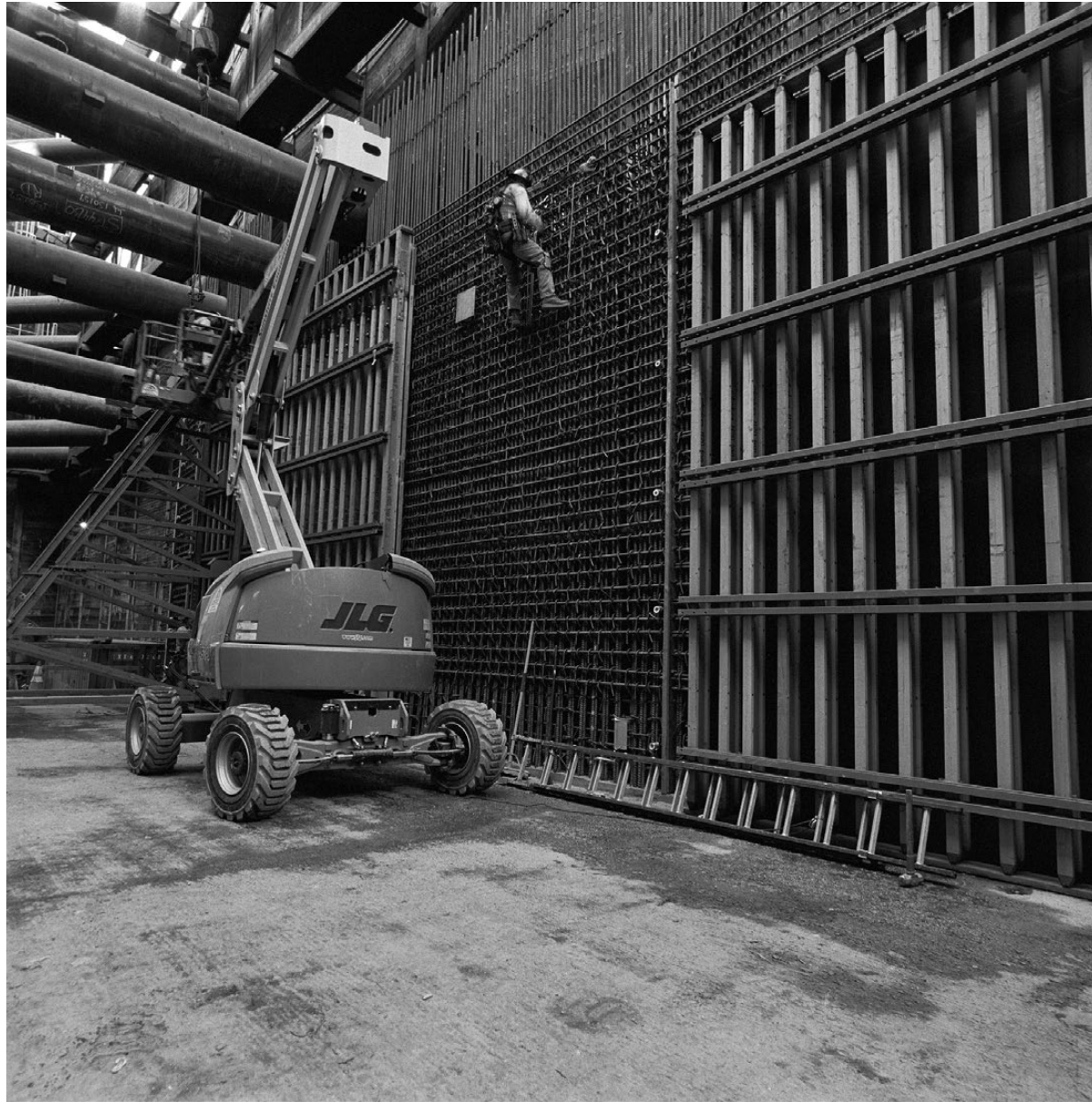
Karagozian shares, "A worker is weaving the rebar to reinforce the new concrete wall being built. Photographing ironworkers walking on the steel is like watching a trapeze artist at work."
