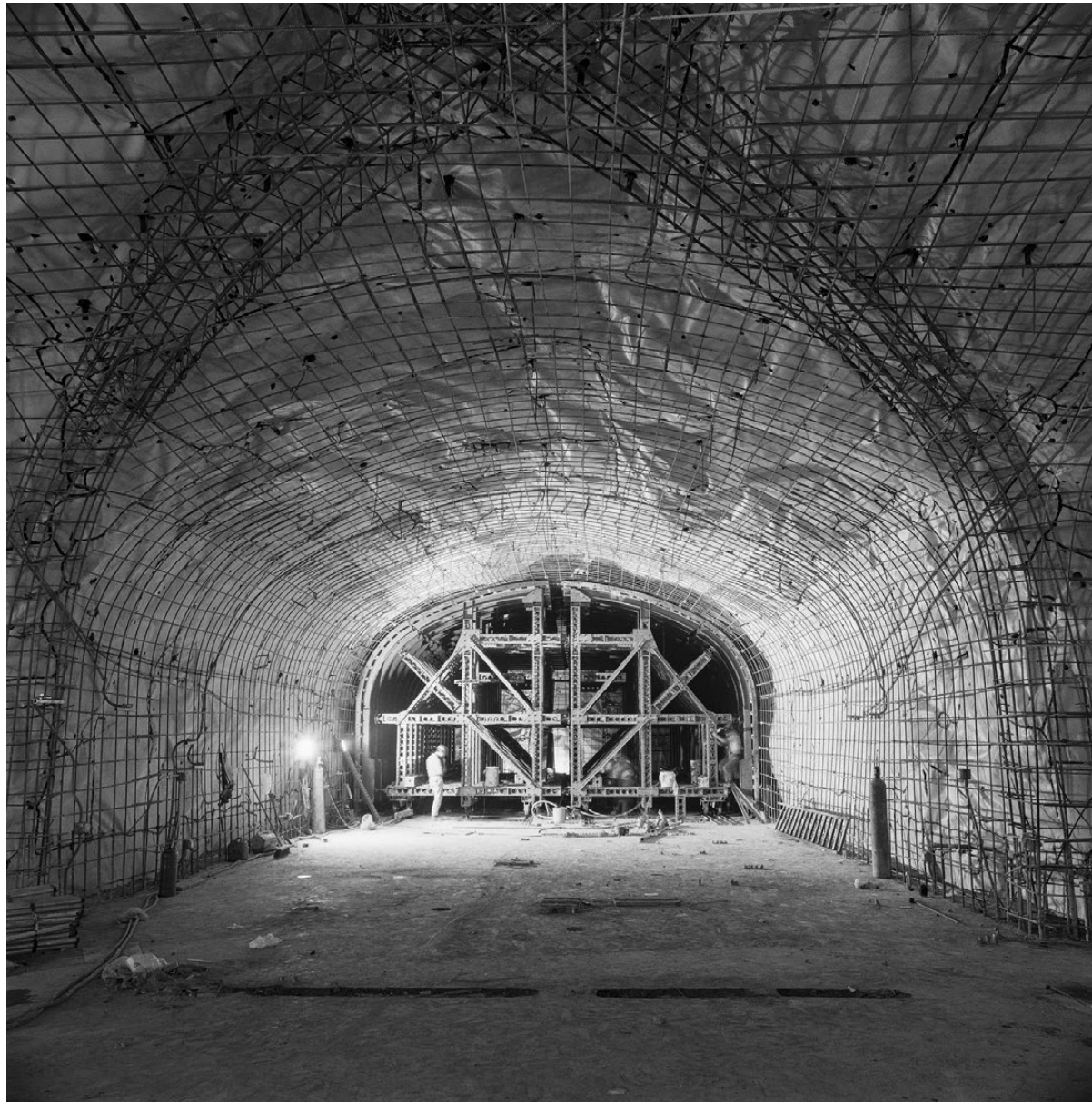
The concrete formwork assembly is shown within the Red Line Track Level Rooms excavated under the Santa Monica Mountains. These rooms house the gear controlling the crossover and the track and power equipment.
