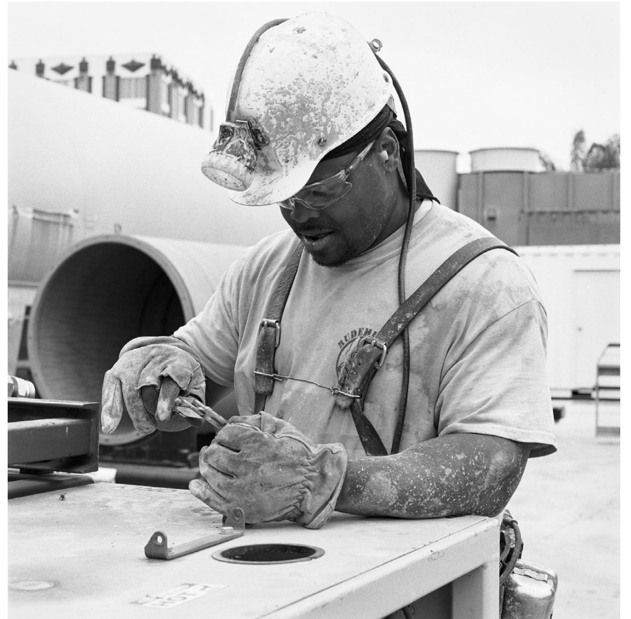
As Karagozian recalls, "I first met Jermaine Hampton, Miner, at the future Little Tokyo/Arts District Station. Here he is working topside (above ground) on the Purple Line Extension Section 1."
