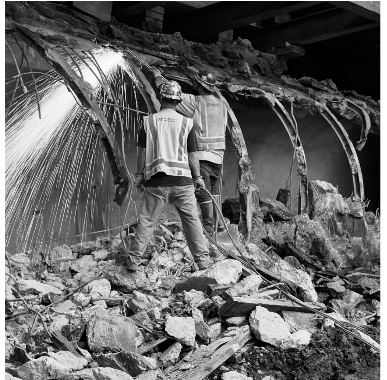
Construction workers dismantle a concrete storm drain under 2nd Street at the future station.
