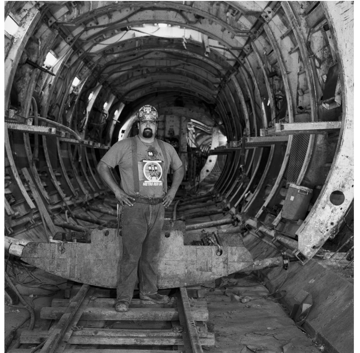
Tony Olea III is standing next to the concrete tunnel arch form for the Red Line. Per Karagozian, Olea III is currently Vice President of the Laborers Local 300 Union and his son is working on the Purple Line Extension.
