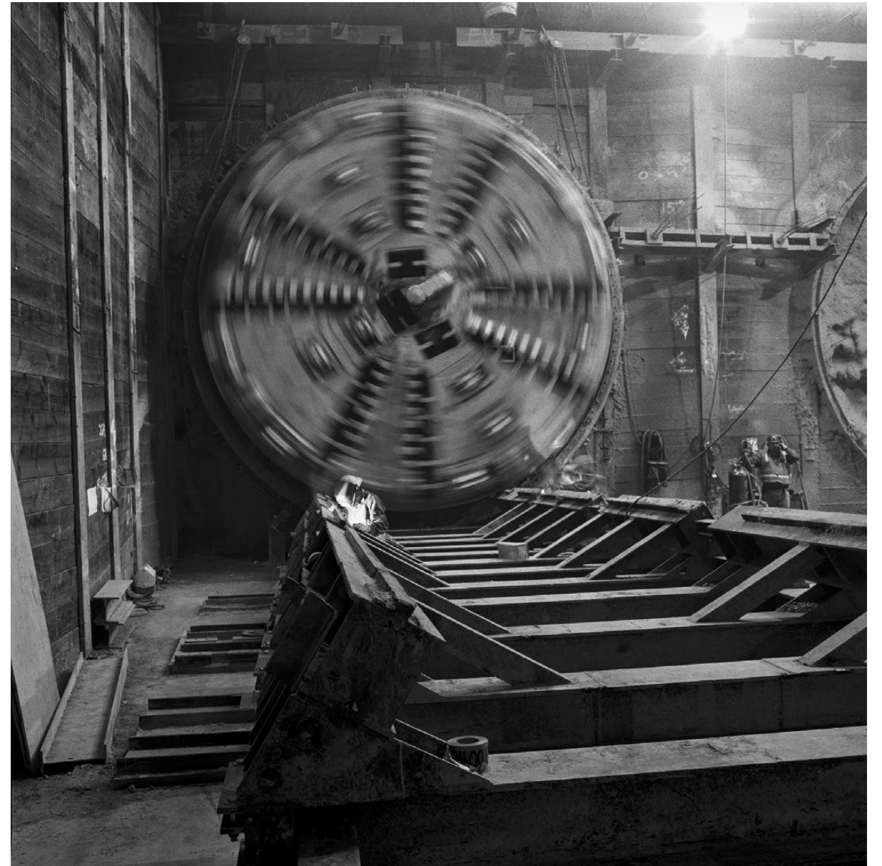
The TBM cutterhead is turning for a press event to showcase the 1.4-mile underground tunnel boring breakthrough in the Gold Line Soto Station. The construction worker is welding the steel cradle for the TBM to be moved onto.
