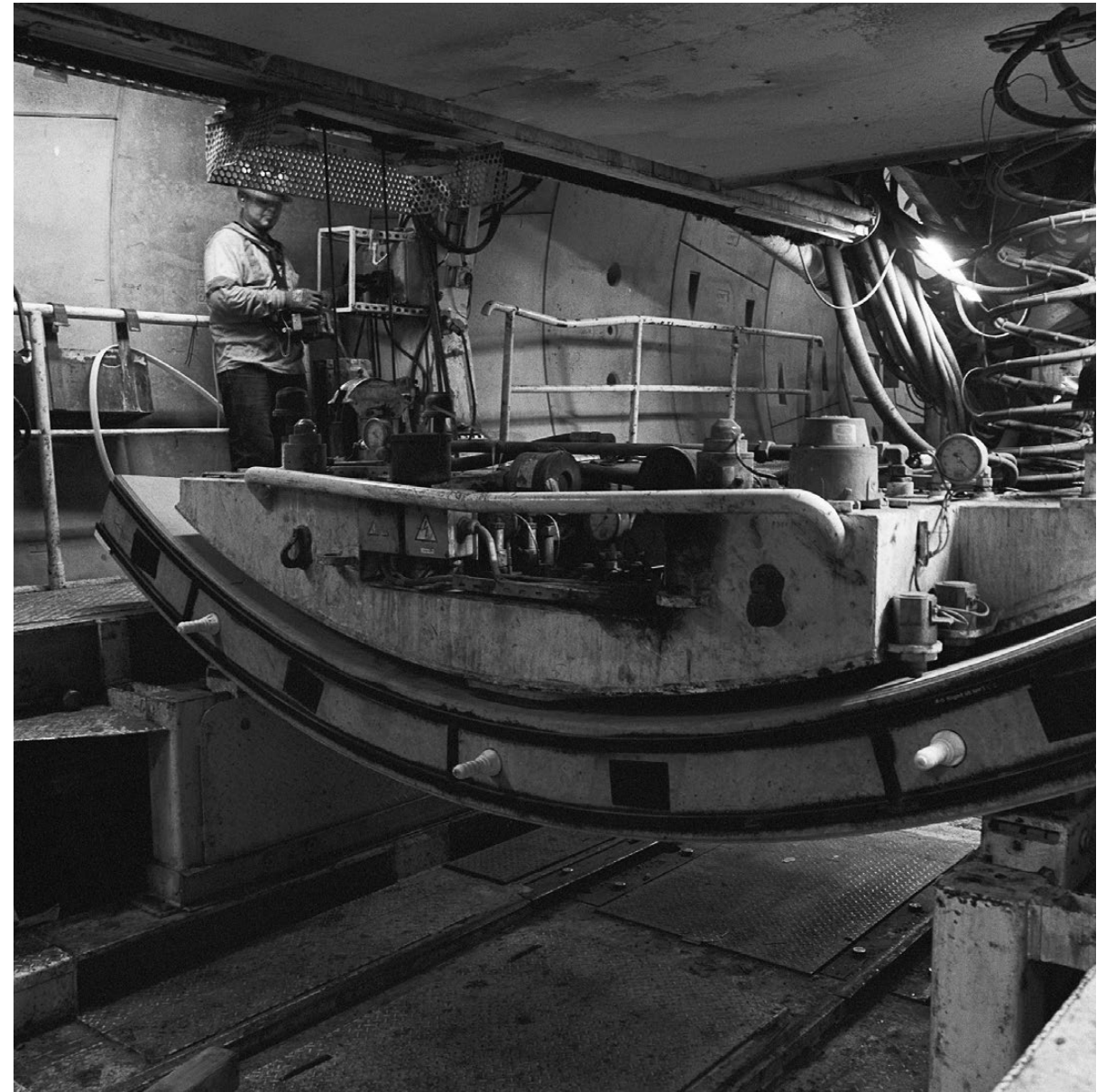
It takes six precast concrete tunnel lining segments to assemble a five-foot wide tunnel lining ring with a 18'-10" inside diameter. Inside the tail shield of the TBM, the operator works the remote control for the vacuum hoist cable crane that transfers the segments into place.
