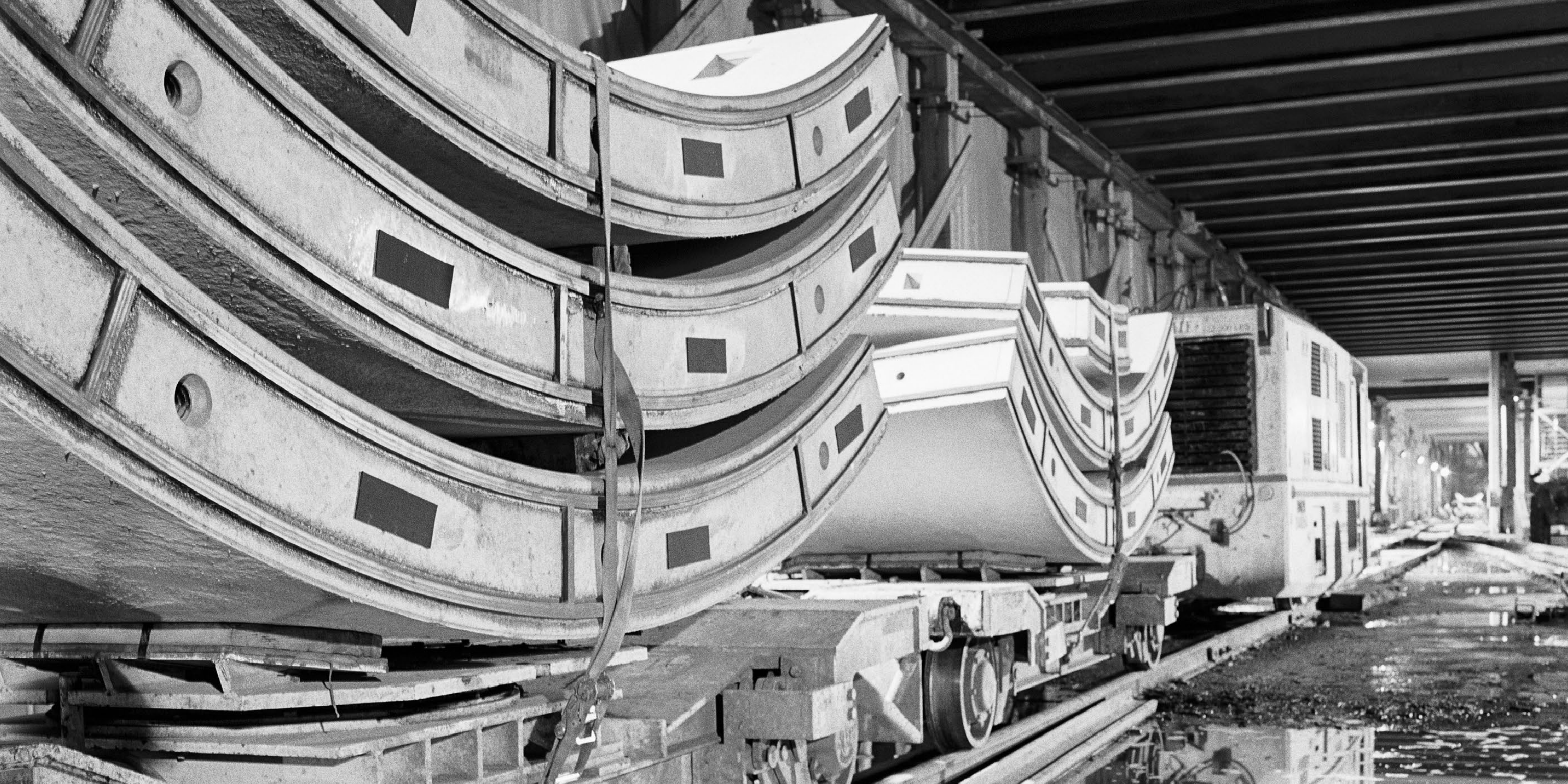
Concrete segment tunnel liners are reflected in puddles of rain water at the bottom landing of the future station. The rail cars deliver these tunnel segments to the TBM.
