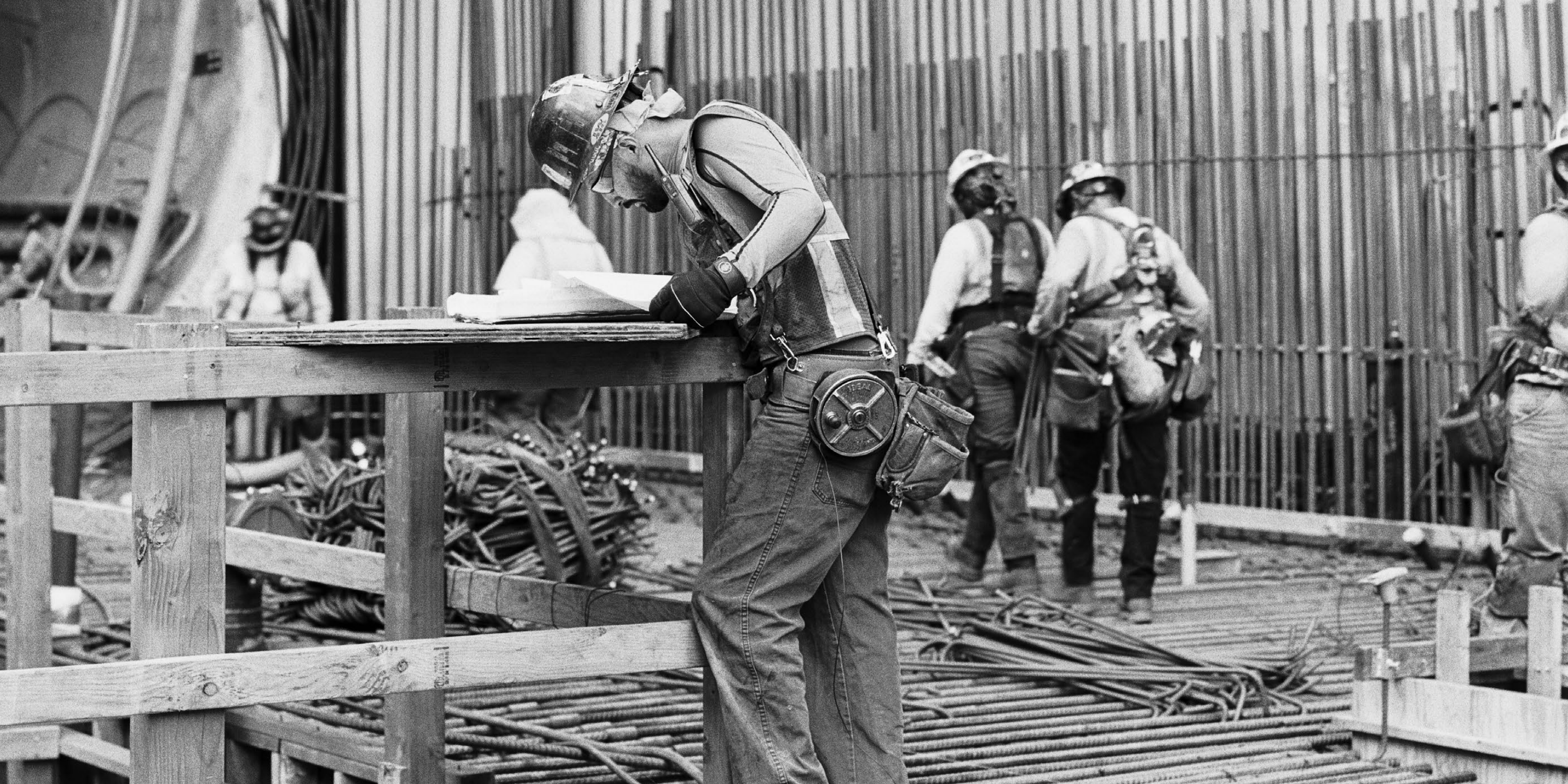
Jorge A. Ocampo, Foreman, looks at the drawings for rebar placement at the future station.
